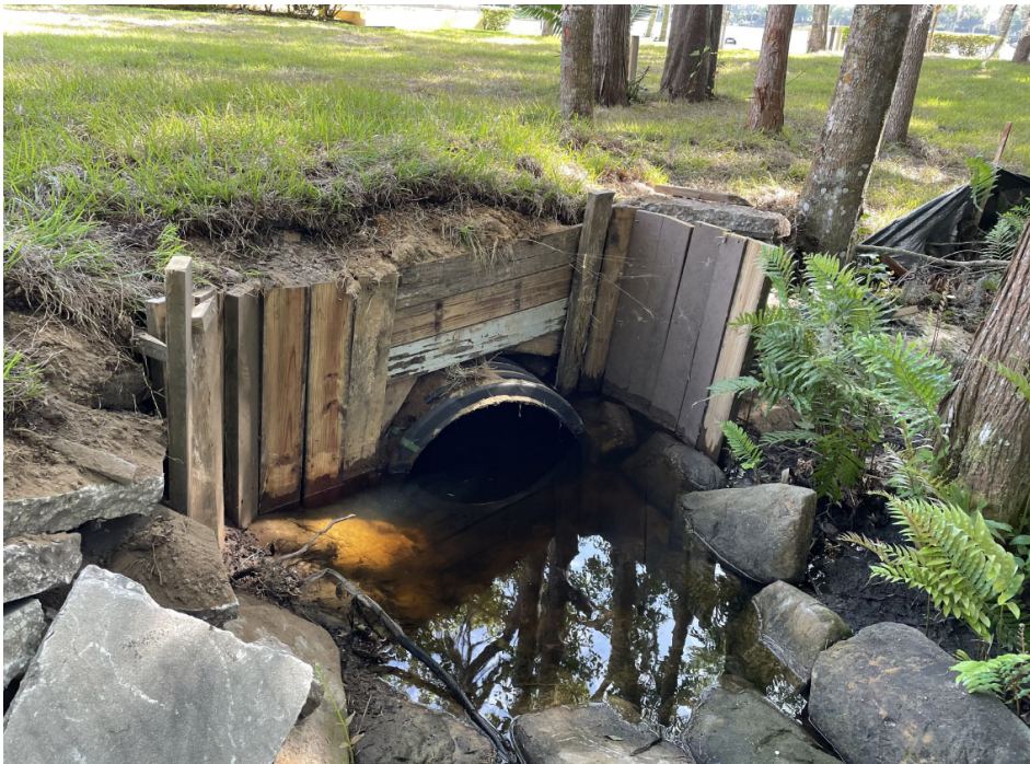
Photo 3 – Homeowner Installed Pipe Directly Discharging into Wetland
